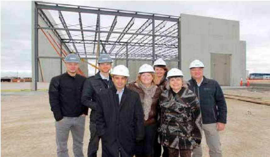
Bird Construction's (from left) Nathan Wiebe and Paul Bergman, Shindico Realty's Robert Scaletta, CentrePort CEO Diane Gray, RM of Rosser Coun. Angela Emms, Rosser Reeve Frances Smee and Bird Construction's Richard Marshall in front of the partially constructed building in CentrePort.
